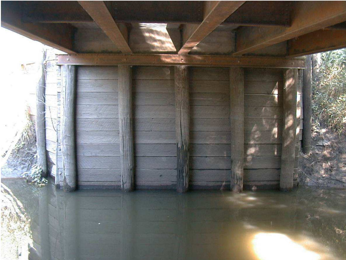
Figure 7.2. KCB2 Pile Deterioration.
