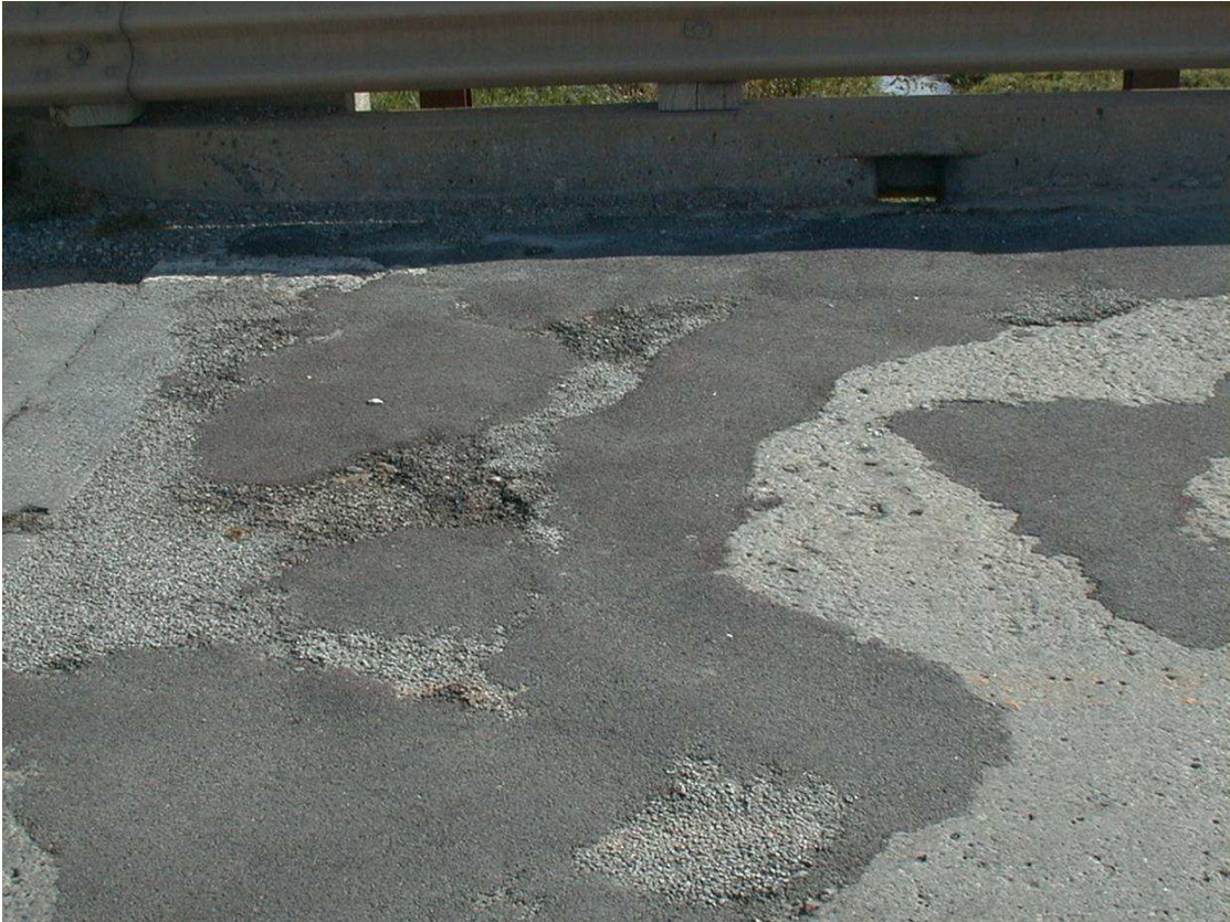
Figure 6.2. Asphalt Patches in CCB Concrete Deck.
