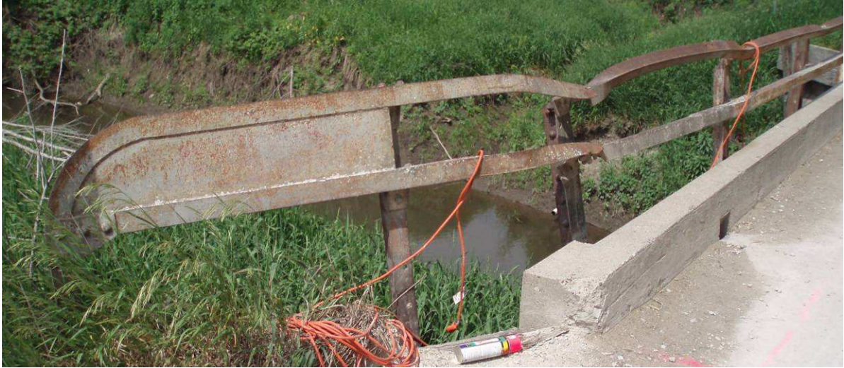
Figure 7.3. KCB2 Railing Damage.
