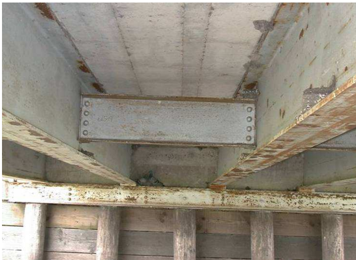
(a) Minor rust on girders
