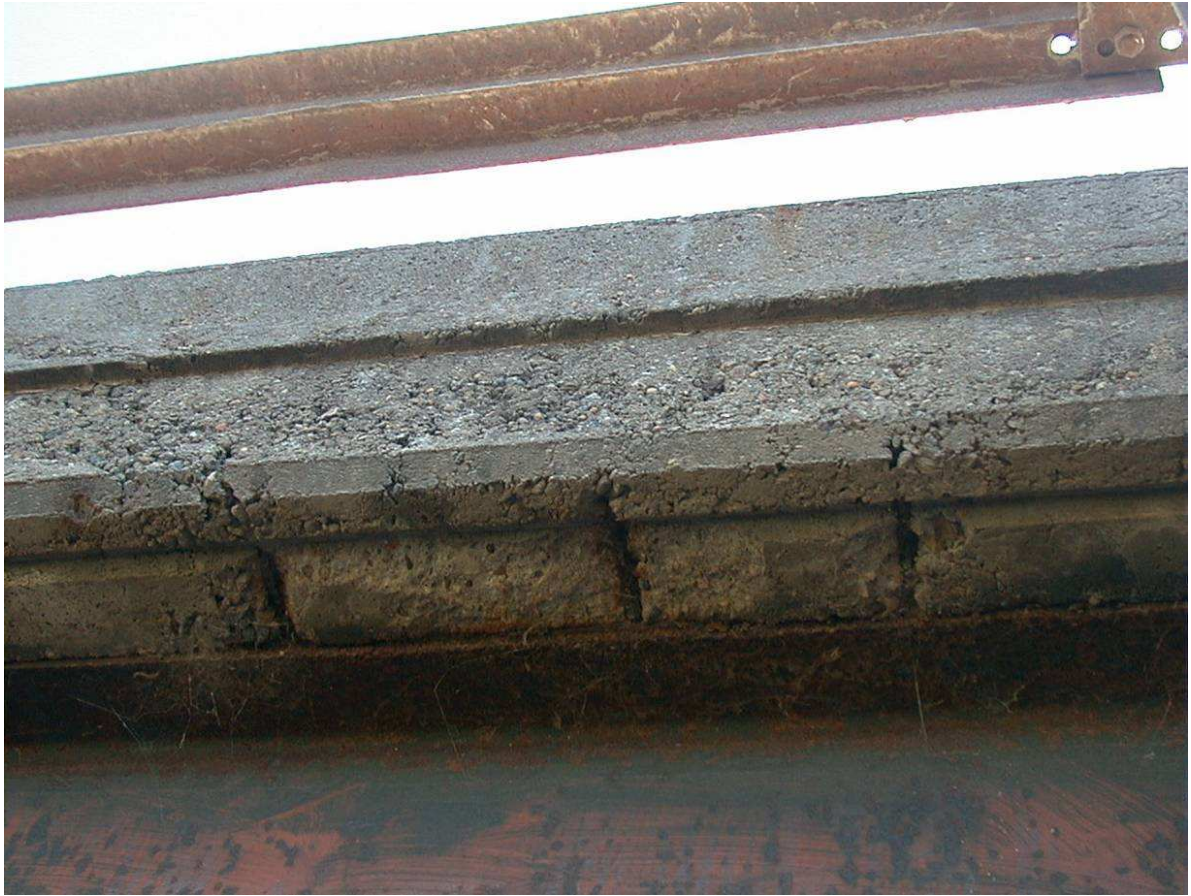
Figure 5.2. KCB1 Poor Concrete Consolidation.
