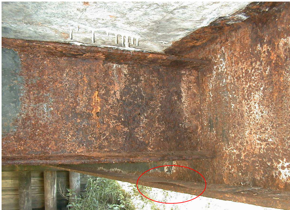
Figure 4.2. MCB Girder 2 Deterioration and Delamination.
